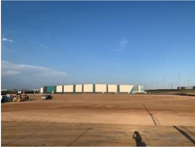
Figure 2: View of subject site looking east from Eastern Creek Road (Source: Mecone)
