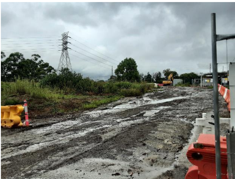
Photo 15 Graded driveway on the western side of the study area, facing south-west
