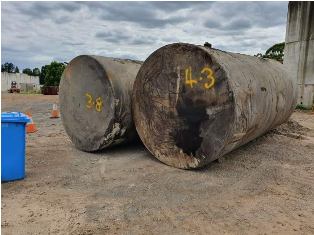
PHOTOGRAPH 7 Condition of removed Tanks 1 & 2.
