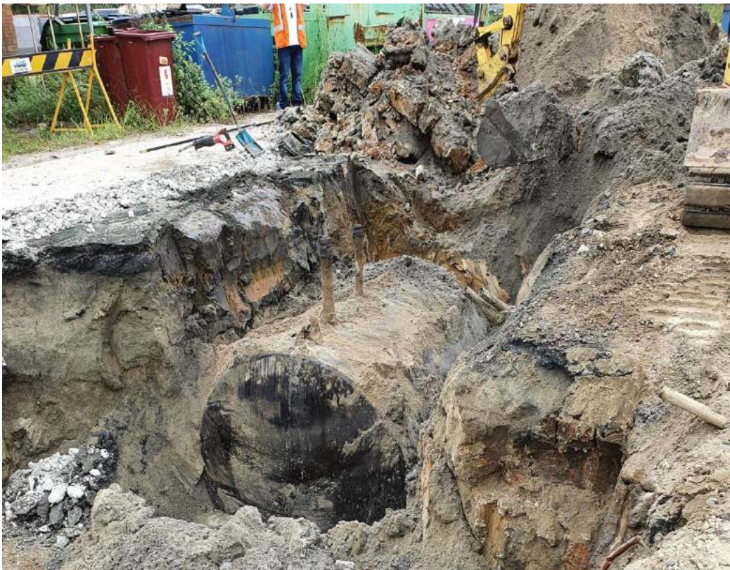
PHOTOGRAPH 2 Black staining on northern wall adjacent Tank 3.
