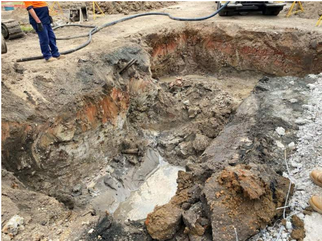
PHOTOGRAPH 6 Groundwater encountered at base of pit excavations.
